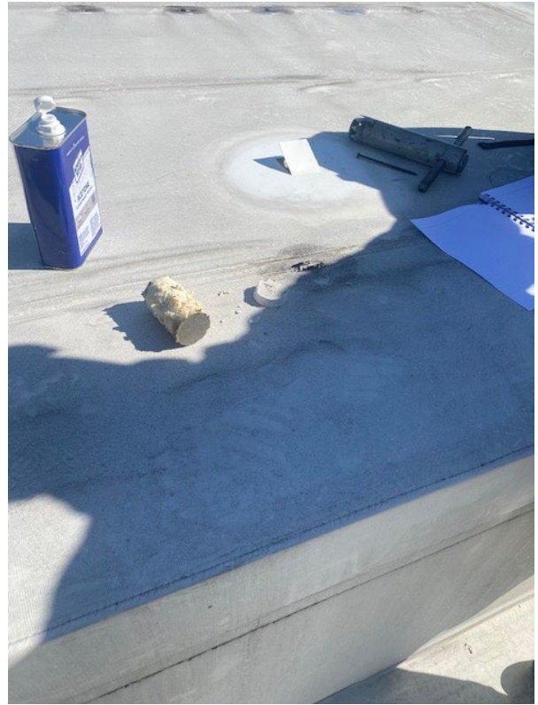
New Roof – North Study Room "Bump out" DuroLast over 3" insulation over 5/8" gyp over metal deck
