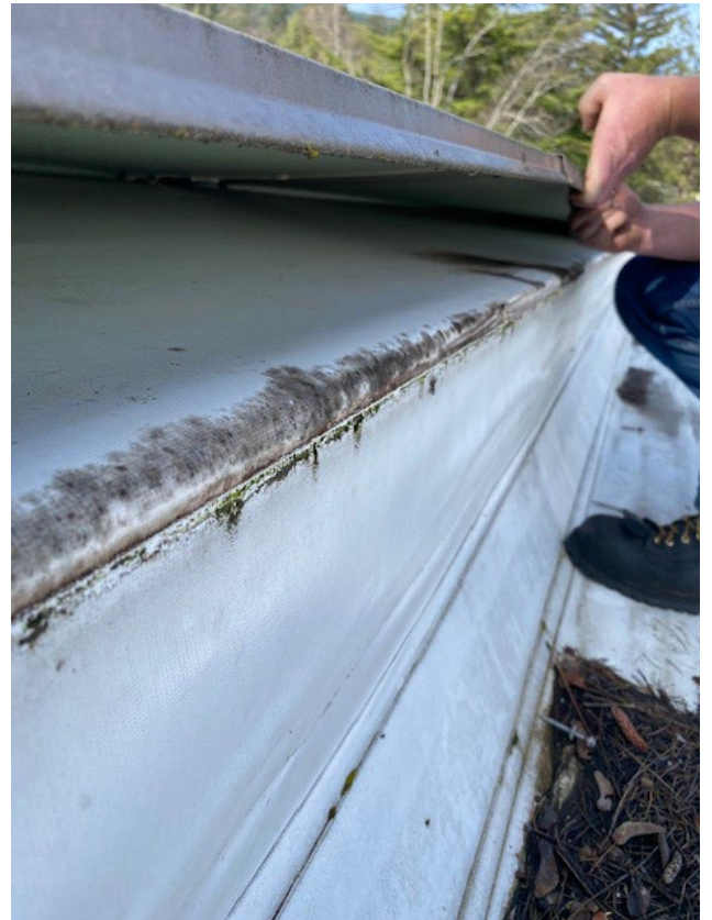
Underside of Coping – Old Roof
