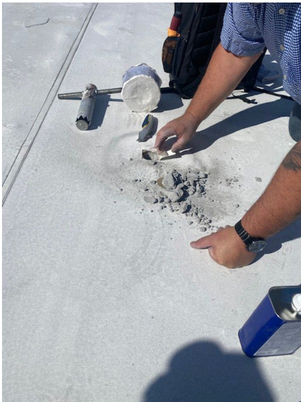
Old Roof – Main Section DuroLast over old membrane over crumbly fill over concrete
