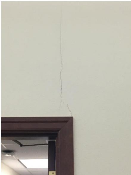
Cracking on the 2 nd floor
