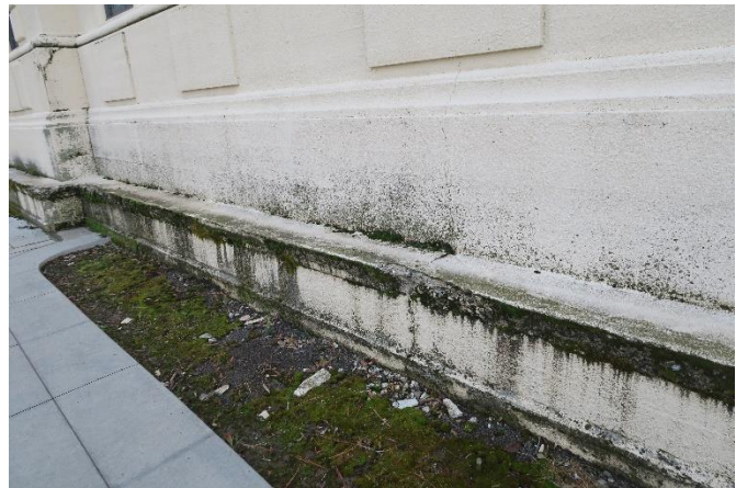
Exterior failure and water intrusion
